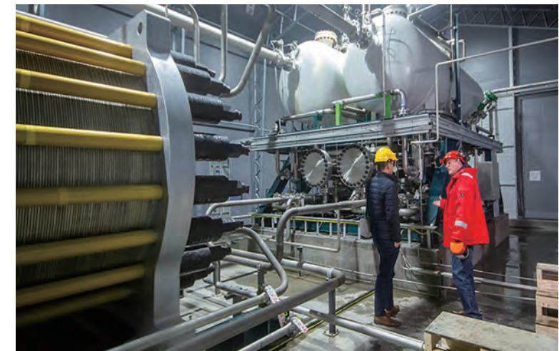
Figure 20 HydrogenPro water electrolysis system
