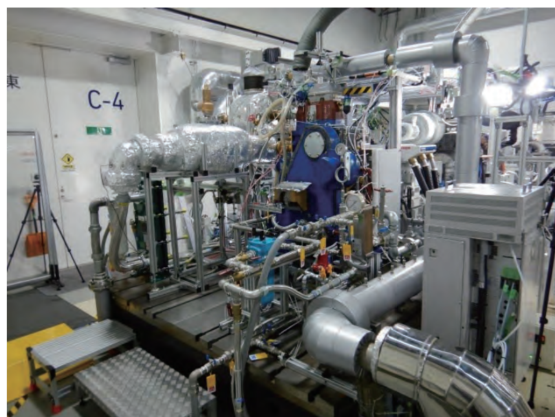
Figure 7 A hydrogen engine installed at the AIST Fukushima Renewable Energy Laboratory
