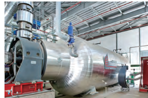
Figure 14 Turboden ORC power generation unit
